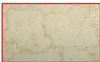
Marbling caused by impurities in steam condensate
