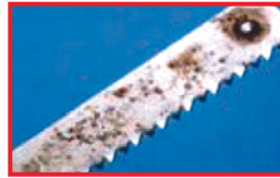
Material affected at partially defective chrome coating. Causes: Humidity causes corrosion to form on unprotected carrier material (normal steel).
