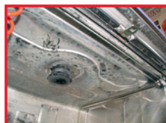
Rinsing chamber with heavy limescale deposits
